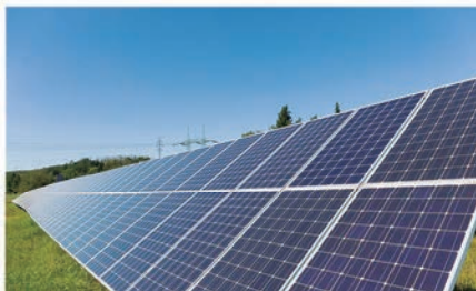
Yuzhou Peak Photovoltaic Power Station Project
